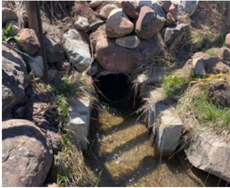
Diversion 1 - 18" culvert with concrete diversion structure with two-way gate.
