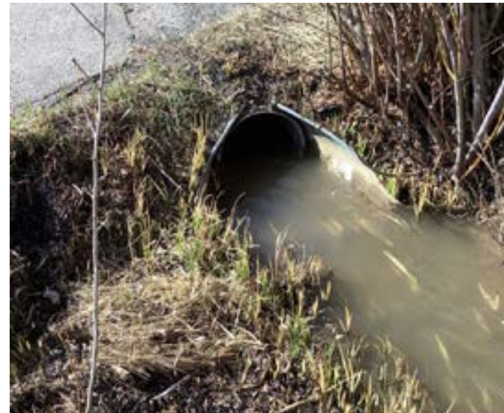
Culvert 15 - 12" culvert with wing-walls directing water under residence driveway (Inflow).
