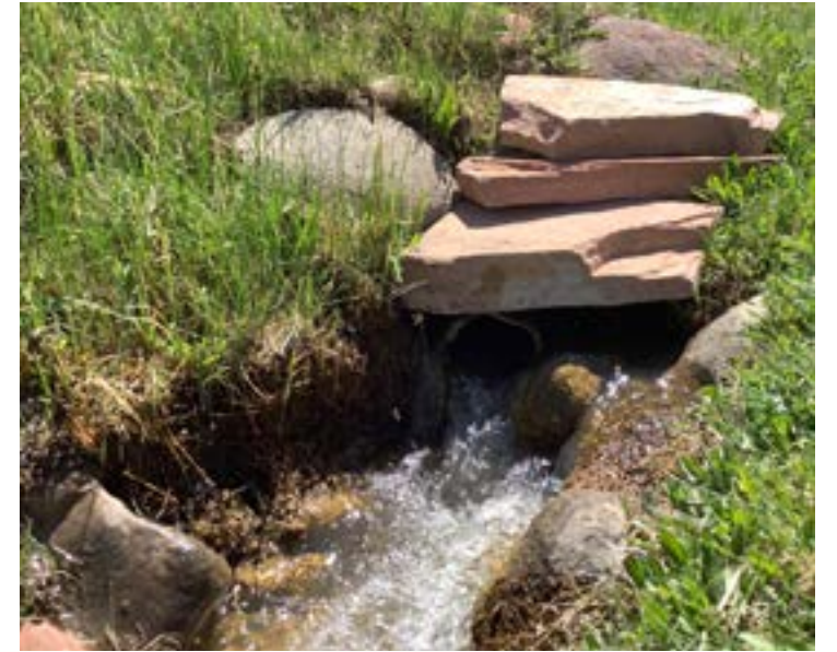
Diversion 12 - No structure, diverts through small 4" pipe.
