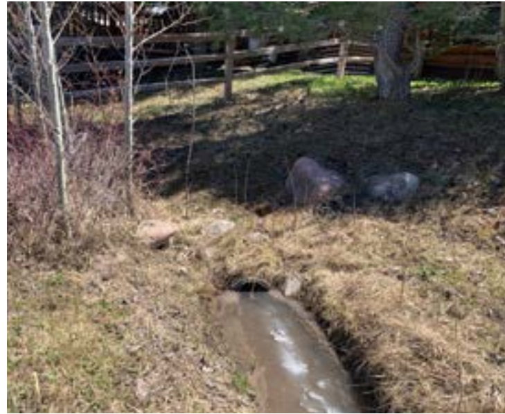
Culvert 3 - 12" culvert, directing water under portion of property landscaping.
