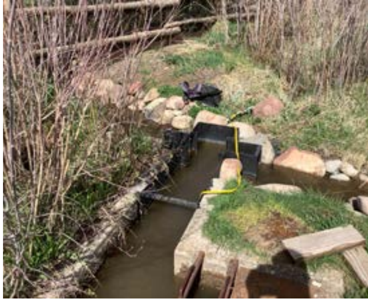
Diversion 17 - Concrete and metal diversion structure with three gates. Two gates divert water to the ponds to the north and south.
