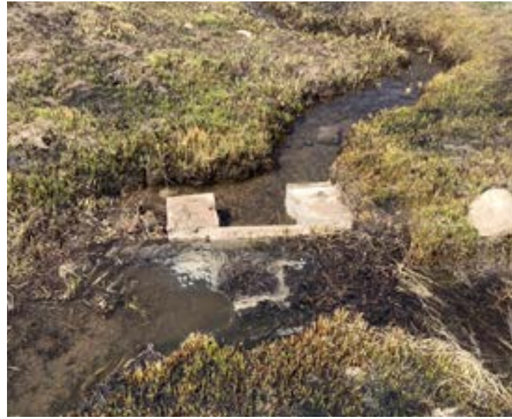
Diversion 2 - Concrete diversion / gate - not working, water flow subverting structure on both sides. Channel measured to be 4', structure is 3'
