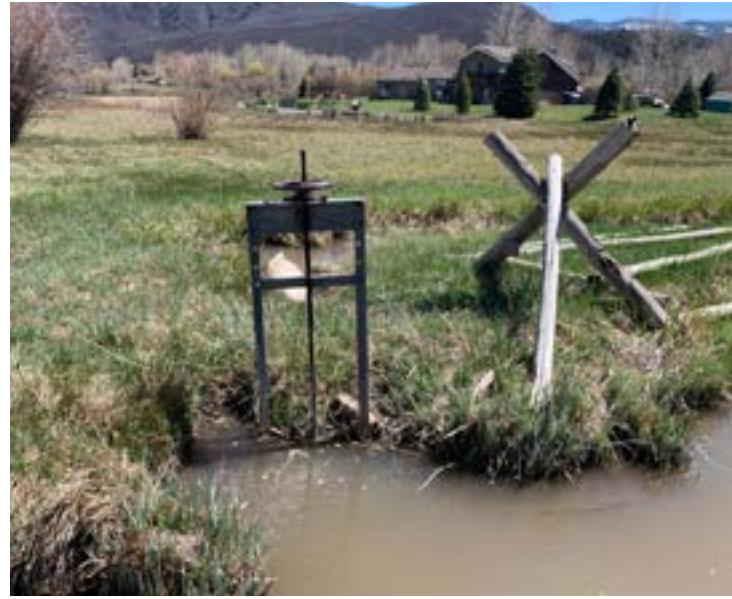
Headgate 2 - Ditch turnout/headgate with 18" outlet.
