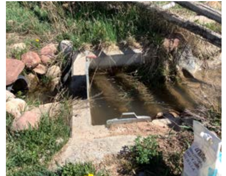
Diversion 16 - Concrete diversion box with two gates with 12" outlets. Structure 3' x 2.5'.
