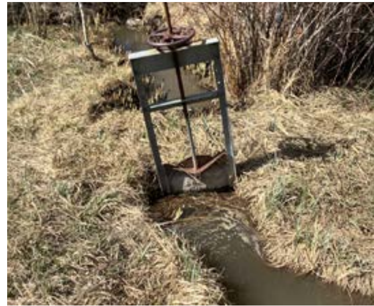
Headgate 7 - Headgate with 15" outlet.
