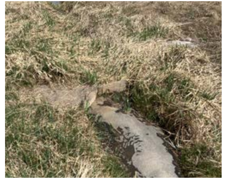
Diversion 8 - Wood boards with concrete foundation and pipe diverting water to smaller ponds. No structure to main ditch/pond.
