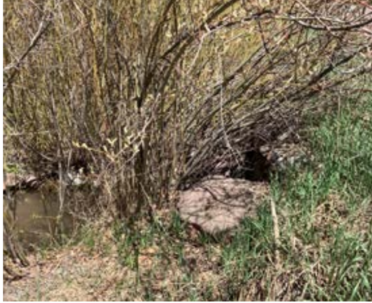
Culvert 17 - 22" culvert directing water under Haystack Lane (Outflow). Limited access due to willows.
