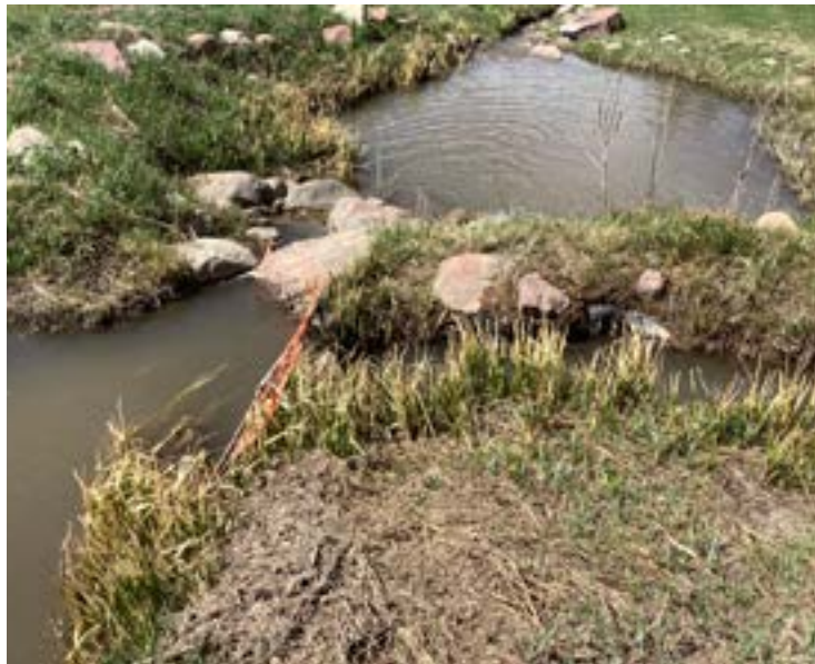
Diversion 13 - Three-way diversion. Concrete structure with 2' opening and boards to control water levels diverting to the west.
