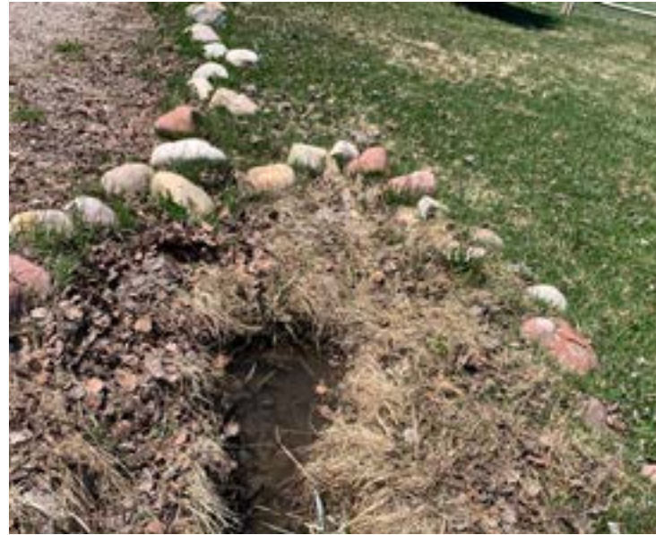
Culvert 2 - 12" culvert, directing water under portion of property landscaping.
