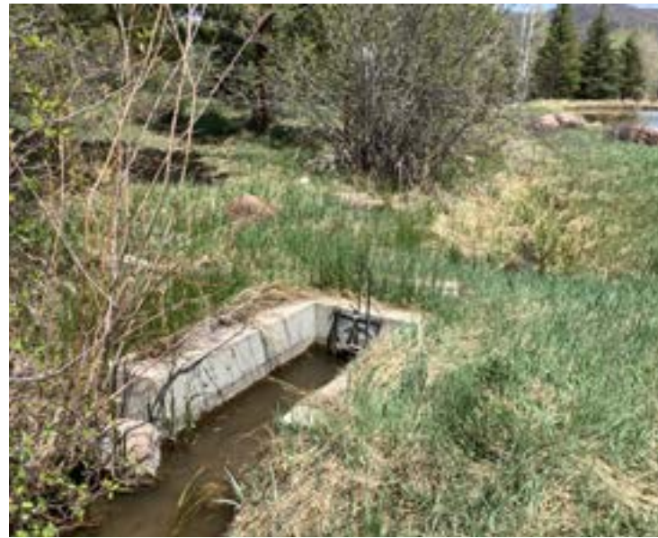
Diversion 6 - Concrete diversion box with two gates. Structure 2'W x 4'L with 10" diversion pipes. Diverts water to upper pond.
