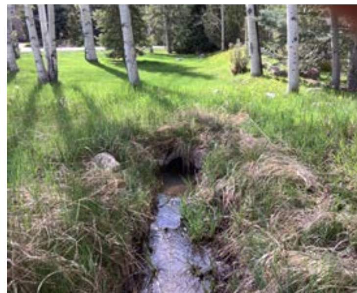
Culvert 23 - 12" culvert directing water underneath Little Elk Creek Ave and through large portion of landscaping.
