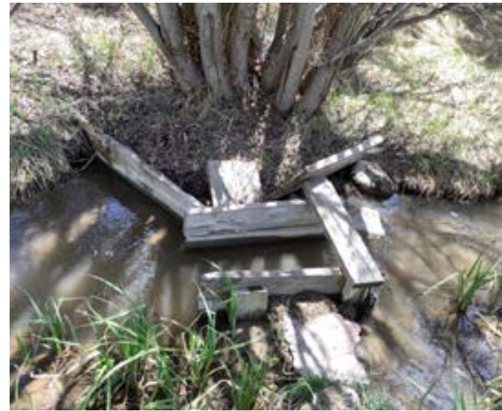
Diversion 7 - Old diversion box constructed of wood material with no gates. In poor condition, likely not functional.
